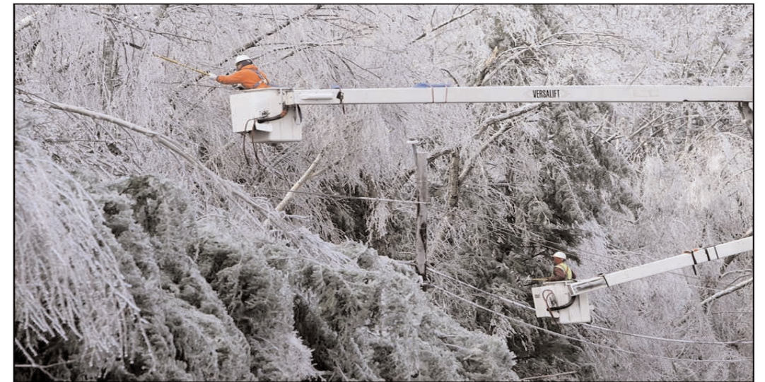
Crews worked to restore power for days after devastating ice storms damaged power lines.
